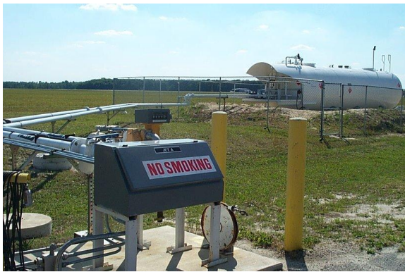
DeCrane's fuel storage system
